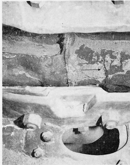
図38 裏面部分写真 矢印で示した亀裂は図36参 照。 Fig. 38 Normal photograph of the inside, a section corresponding to the scope of X-ray photograph L 17.
